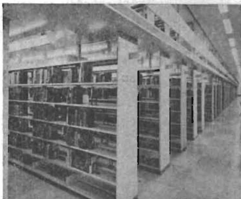
Multi-tier bookstacks and mezzanine cellular decking installed in September, 1964 at University of Victoria, B.C. Mr. Dean W. Halliwell, Chief Librarian. R. W. Siddall Associates, Victoria, B.C., Architect
