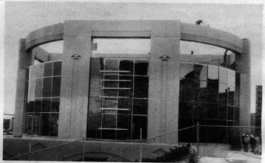
Construction continues on "Alderney Gate" which will house the new Dartmouth Regional Library.
